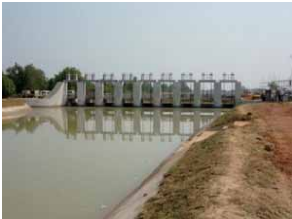
Main Canal and Cross Regulator, Rengali Irrigation Sub-Project (L.B.C-II, Phase-I), India, with JICA Loan
