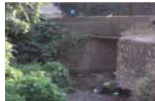
Korbou Bridge- Overflow during heavy rain (Before the Project)
