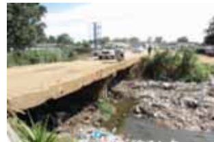
Mudarat Bridge - Old and narrow bridge (Before the Project)
