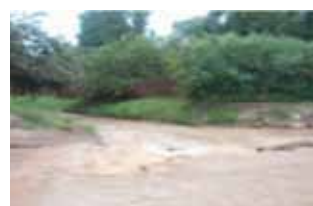
Culvert No.15 - Flooded during heavy rain (Before the Project)
