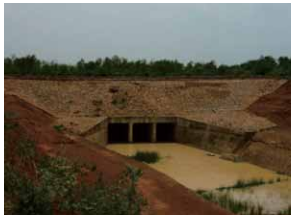
Elephant Corridor across Main Canal, Rengali Irrigation Sub-Project (L.B.C-II, Phase-I), India, with JICA Loan
