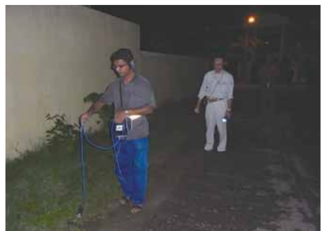
OJT for leak detection in a pilot area
