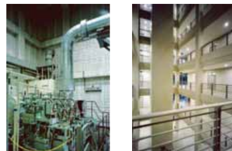
Real Diesel Engine Plant and Lobby Atrium: BP3IP Jakarta
