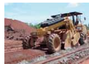
Section 6, Stabilization, stabilizer
