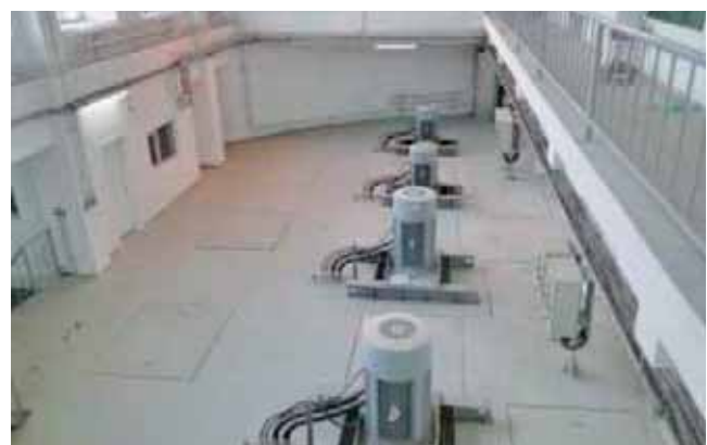
Discharge Pump Station
