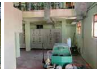
Pilot project for algae removal by Micro-strainer
