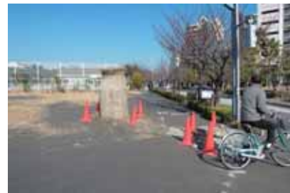
Uplifted manhole by liquefaction Photo: Nihon Suido Cosultants
