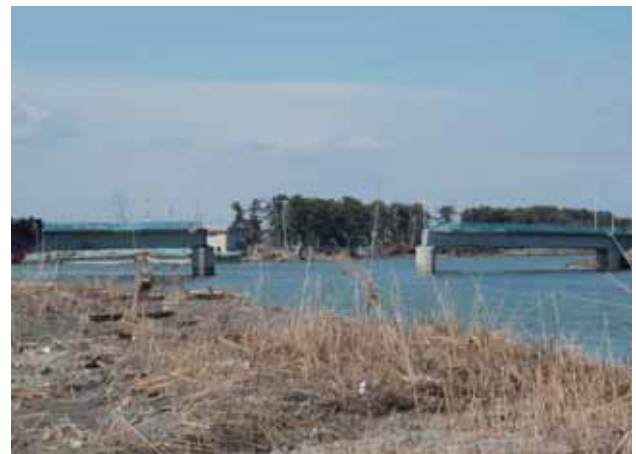
Center bridge girder was taken away by Tsunami Photo: Oriental Consultants
