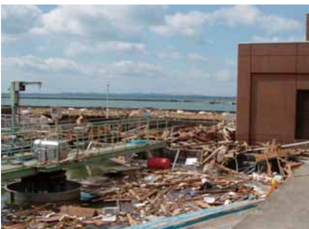
Sewage treatment facility blocked by a heap of rubble
