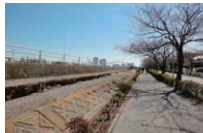
Bumped seawall caused by liquefaction Photo: Chuo Kaihatsu
